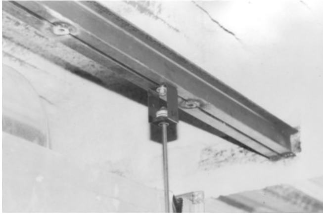
Figure 7-5 Overloaded spring hanger.
