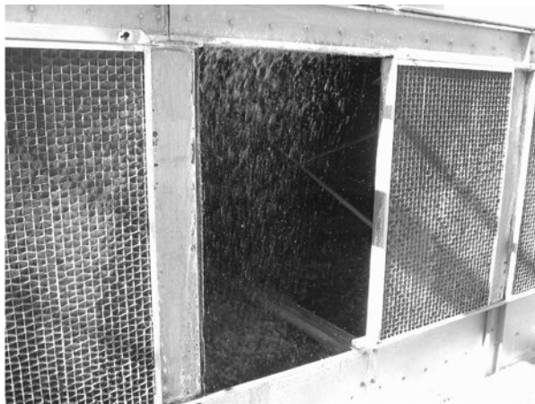
Figure 3-8 Cooling tower basin with free-falling condenser water.
