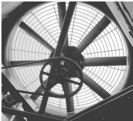
Figure 3-5 View of “standard” cooling tower induced-draft fan.
